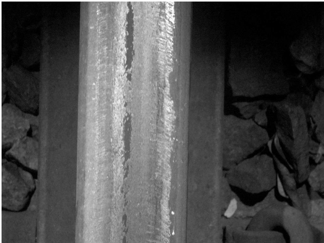
Figure 10 – Typical sample for spalling class.
