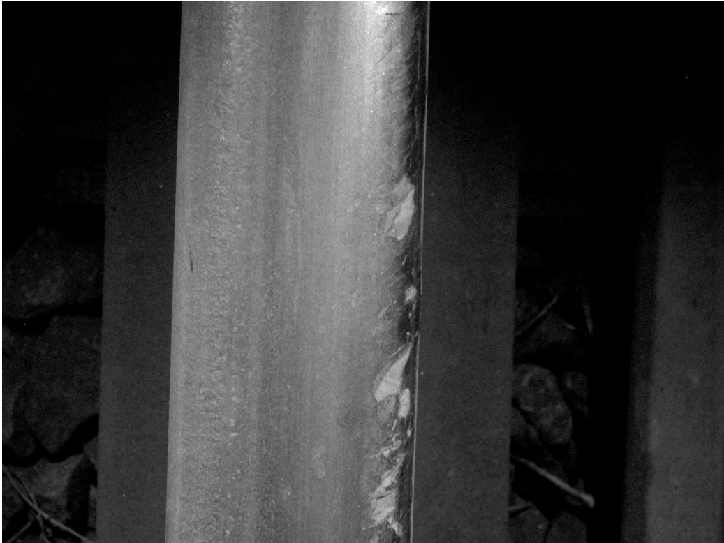
Figure 7 – Typical sample for cracking class.
